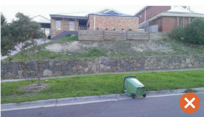
Multi-layered retaining walls with excessive batters towards the street
